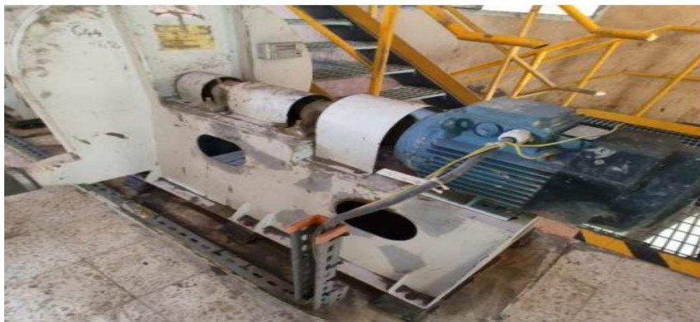
Figure 8. Centrifugal Blower OF AIR-SLID in the packing system of cement factories
