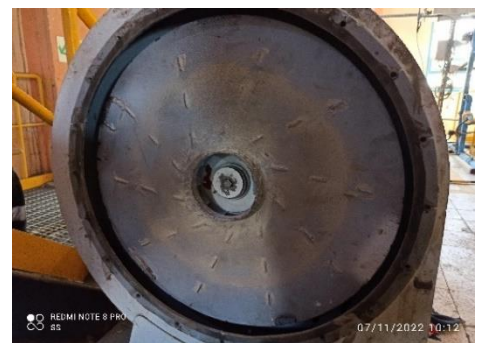
Figure 11. Fan after cleaning
